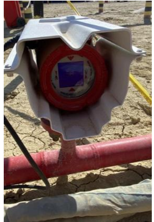
Red Eye hydrate guard meter installation at MEG injection point.
